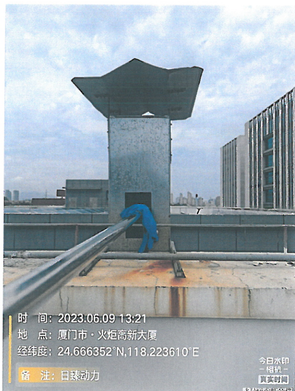
DA001 废气排气筒出口 A#
